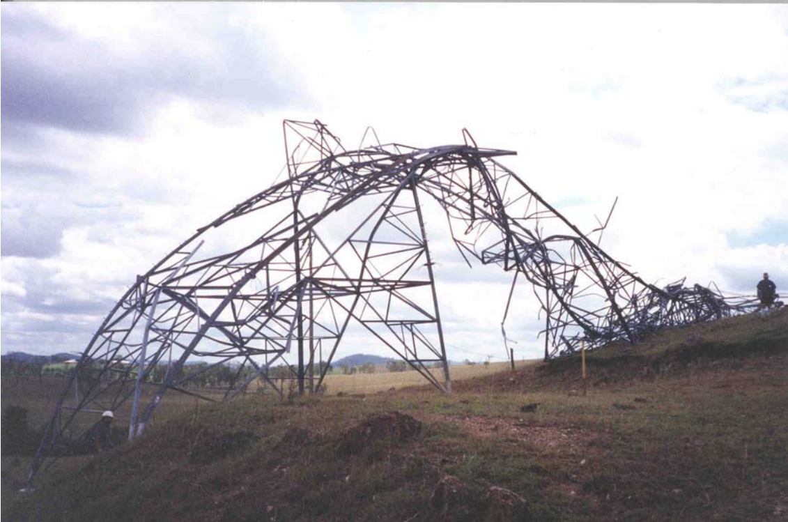
Fig. 1-1 - Damaged transmission tower (275 kV double circuit electricity transmission tower) in the Brisbane valley in March 1998 (Courtesy of Prof C. LETCHFORD)
