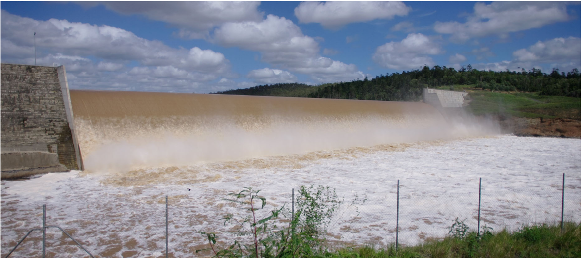
Figure 1. Paradise Dam stepped spillway operation on 5 March 2013 for Q = 2,326 \text{ m}^3/\text{s} and d_c/h = 2.8 (skimming flow regime) (Photograph H.Chanson).
