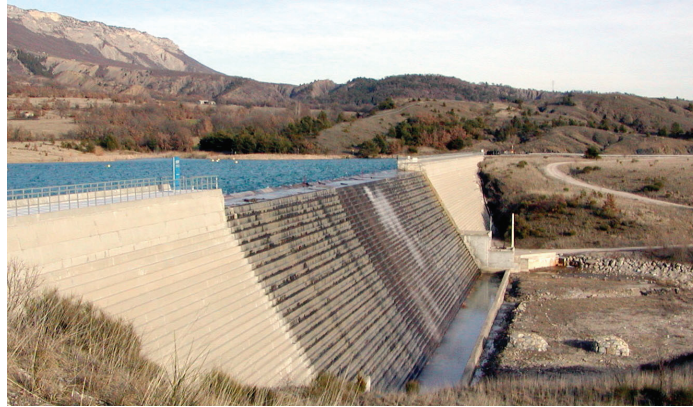
Figure 1. Concrete gravity dam stepped spillway: Riou Dam (France) in 2004, h = 0.43 m, 1V:0.6H slope.
