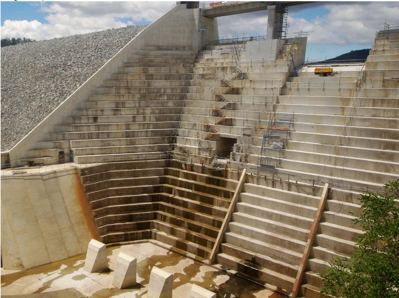
Fig. 1 - Photograph of the Hinze dam stepped spillway (Australia) shortly before completion (Courtesy of SEQ Water)
