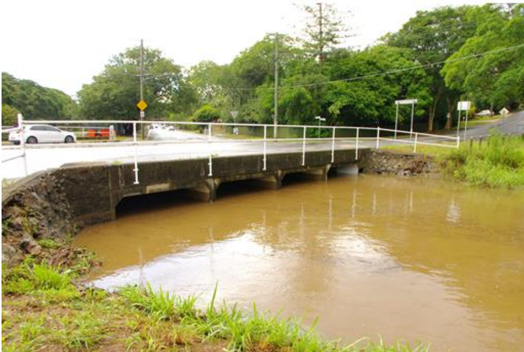
Figure 1. Outlet of multicell box culvert along Witton Creek (Indooroopilly QLD, Australia) on 18 March 2019 after a 40-mm rainfall storm. Looking upstream.
