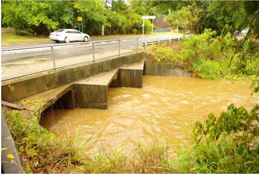
Figure 1. Outlet of multicell box culvert along Witton Creek (Indooroopilly QLD, Australia) on 18 March 2019 after a storm. Flow direction from left to right.
