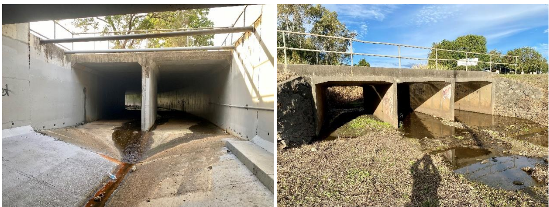
Figure 1. Standard box culvert structures. Left: outlet of 2 cells box culvert on Cubberla Creek, Kenmore QLD (Australia); Right: outlet of multicell box culvert along Coolaba Creek, Yeerongpilly QLD (Australia)
