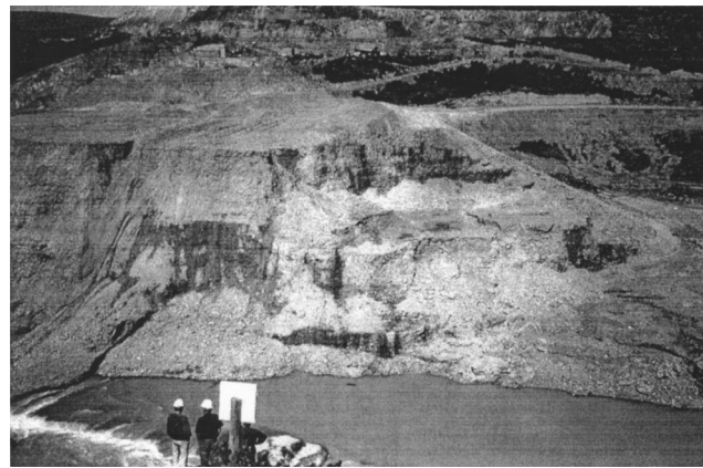
Fig. 2. View from left abutment looking across breach in Opuha Dam toward remaining part of embankment
