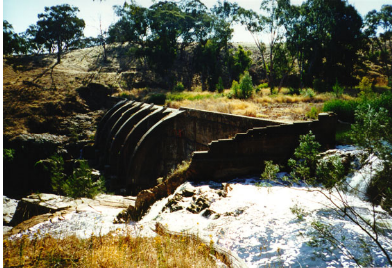
Arch Dams, Development from Cut-Stone Arches to Modern Design, Figure 7 Junction Reefs dam (Lyndhurst NSW, Australia) (Photograph taken on December 28, 1997) View from the left bank.
