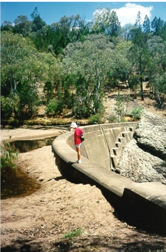
Reservoir Sedimentation in Australia under Extreme Conditions, Figure 2 Dry reservoir of Koorawatha weir, railway dam completed in 1911 – view from the right bank in December 1997.
