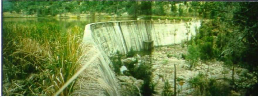
Reservoir Sedimentation in Australia under Extreme Conditions, Figure 5 Fully silted reservoir of Old Quipolly dam (Werris Creek NSW) completed in 1932 – view from the right bank in June 1997.
