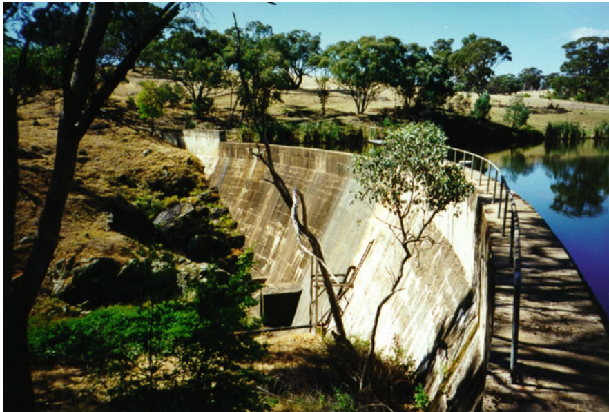
Reservoir Sedimentation in Australia under Extreme Conditions, Figure 4 Borenore Creek dam completed in 1928 – view from the left bank in December 1997. Note the old scour outlet system and the new water intake at half-height of the dam wall.
