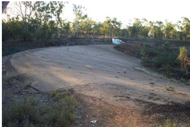
(A) Sandy Creek weir, Clermont QLD during construction in Sept. 2002 (Courtesy of Keith JAMES) - View from the right bank
