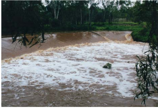
(A) Sandy Creek weir, Clermont QLD on 8 March 1993 (Courtesy of A.J. HOLMES) - View from the right bank
