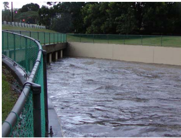
(B) Minimum Energy Loss culvert in Brisbane - Outlet operation on 31 Dec. 2001 for about 80 \text{ m}^3/\text{s} , looking from right bank
