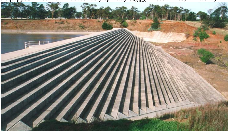
Fig. 2-3 : Melton dam secondary spillway on 30 January 2000 - Completed in 1916, the Melton dam was equipped in 1994 with a secondary spillway ( Q_{des} = 2,800 \text{ m}^3/\text{s} , h = 0.6 \text{ m} )
