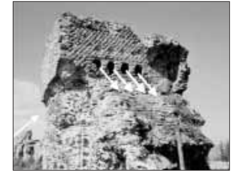
The upstream reservoir of a siphon of the Gier aqueduct: of the ten holes from where the lead pipes departed, four can be seen on this picture. The white arrows show the direction of the flow (photo P.L. Viollet).
