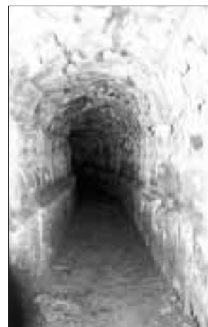
Fig. 2 - Brévenne aqueduct (Lyon, Fra.) at Biternay - Inside view of the subterranean conduit, looking upstream
