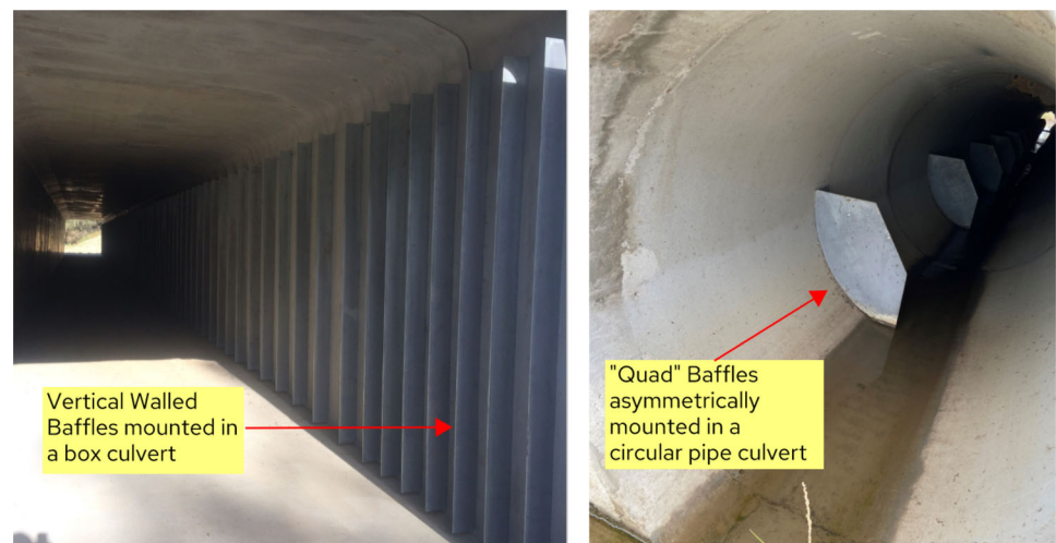
FIGURE 1 Box culverts in Australian fish mapped waterways (Ensilon Consulting, 2024). (LEFT) 3.0 m × 3.0 m reinforced concrete box culvert (RCBC) cell fitted with full-height vertical wall fish baffles at Flagstone, Queensland, Australia. (RIGHT) “Quad” fish baffles fitted to a 1.05-m-diameter reinforced concrete pipe (RCP) at Walloon, Queensland, Australia. For further details on “Quad” fish baffles refer to Kapitzke (2010). [Color figure can be viewed at wileyonlinelibrary.com ]
